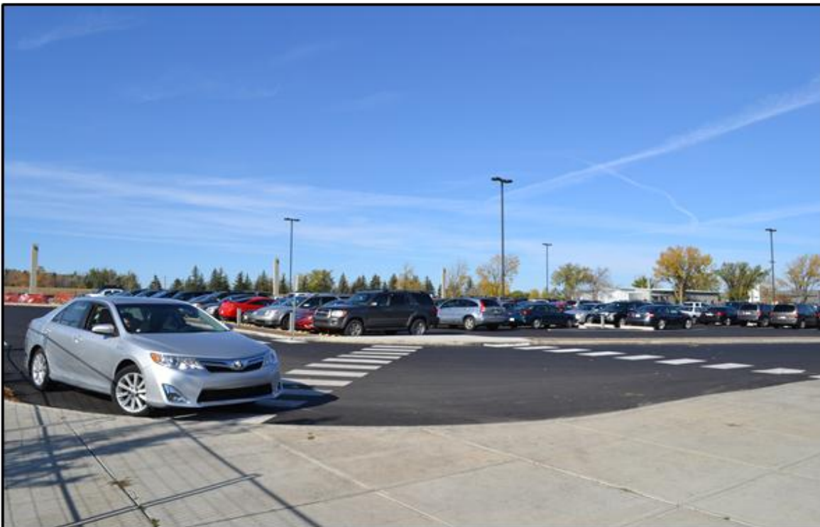
A significant redevelopment of the western parking lots saw the construction of storm water management systems, as well as newly paved roadways and a new entrance to Lot E.
